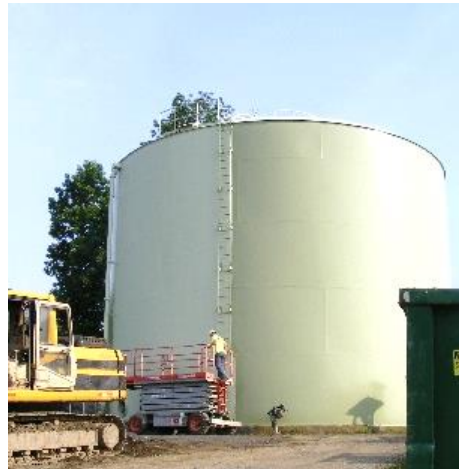
Water Tank / Gallons
