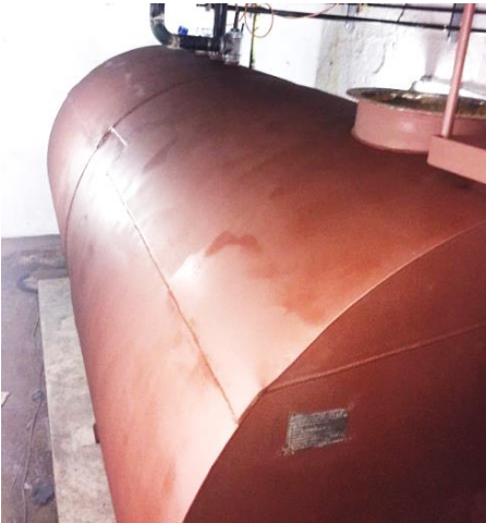
Oil Tank / Gallons
